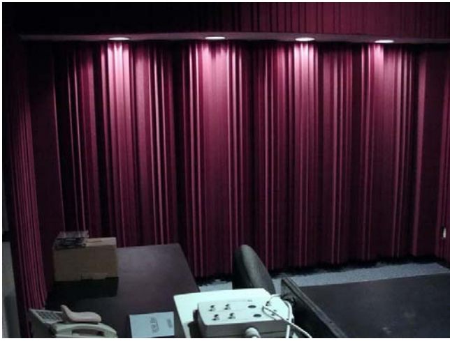
Sunburst Male Broadband Absorbers installed on the back wall of one of the Auralex studios. Consider doing this to a wall or your studio, iso room or iso booth for excellent low-frequency control.
