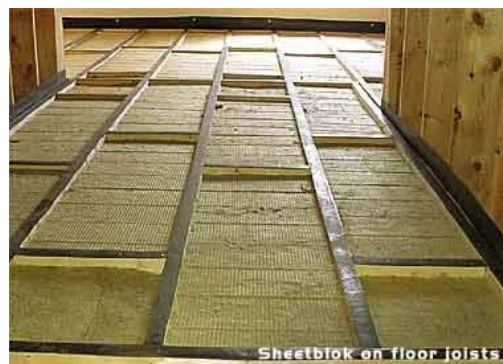
The right way to build a floor by following the Auralex system. Even if you can't build a new floor, though, there are effective steps you can take.
